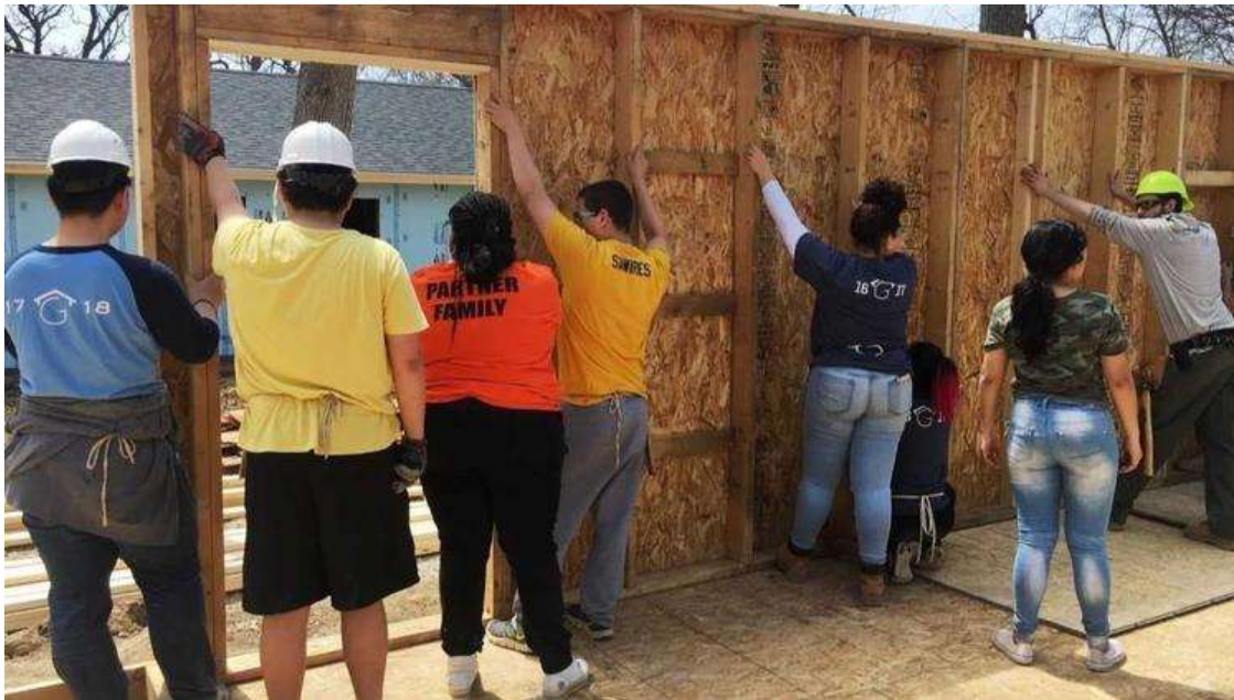
A Glenbrook South High School class that combines mathematics and construction built the exterior and interior walls for a Habitat for Humanity Lake County home in Waukegan and then installed them May 2, 2018. (Habitat for Humanity)
